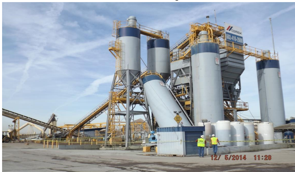
After silo collapse.
