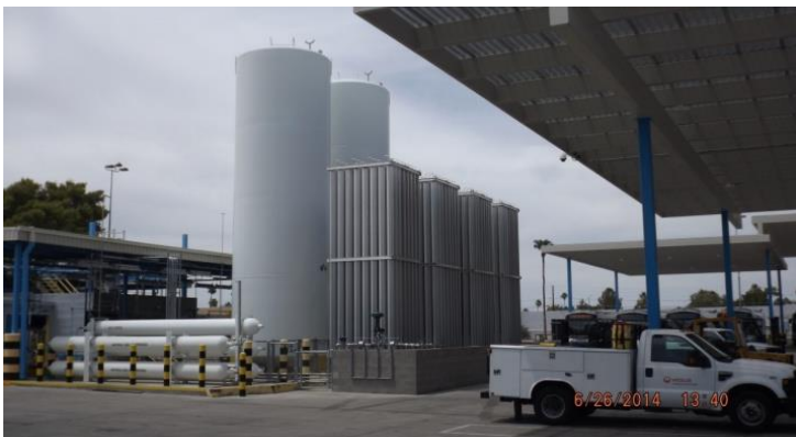
CNG tanks for new buses
